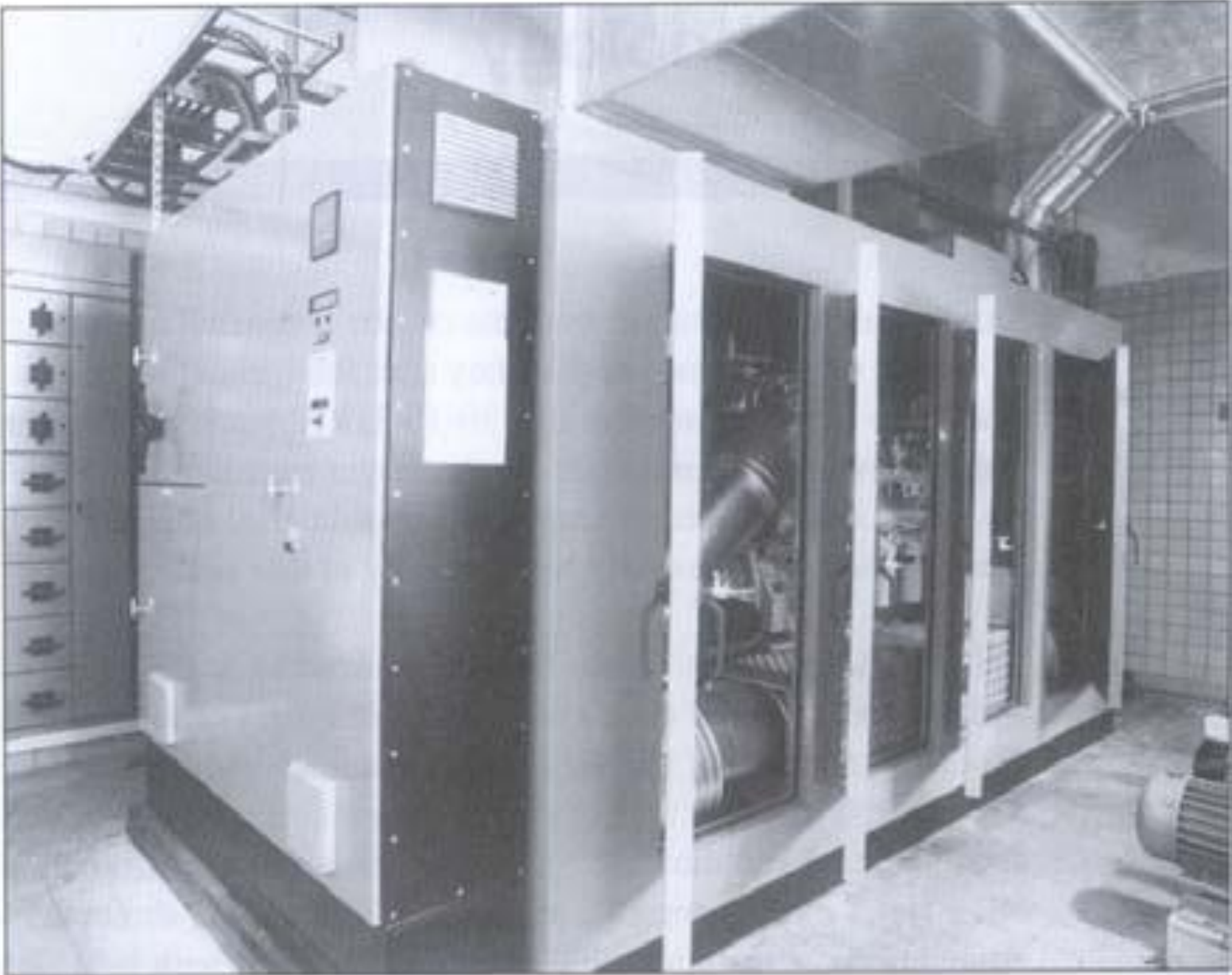
Packaged gas engine cogeneration unit (courtesy of Geveke Motoren).
